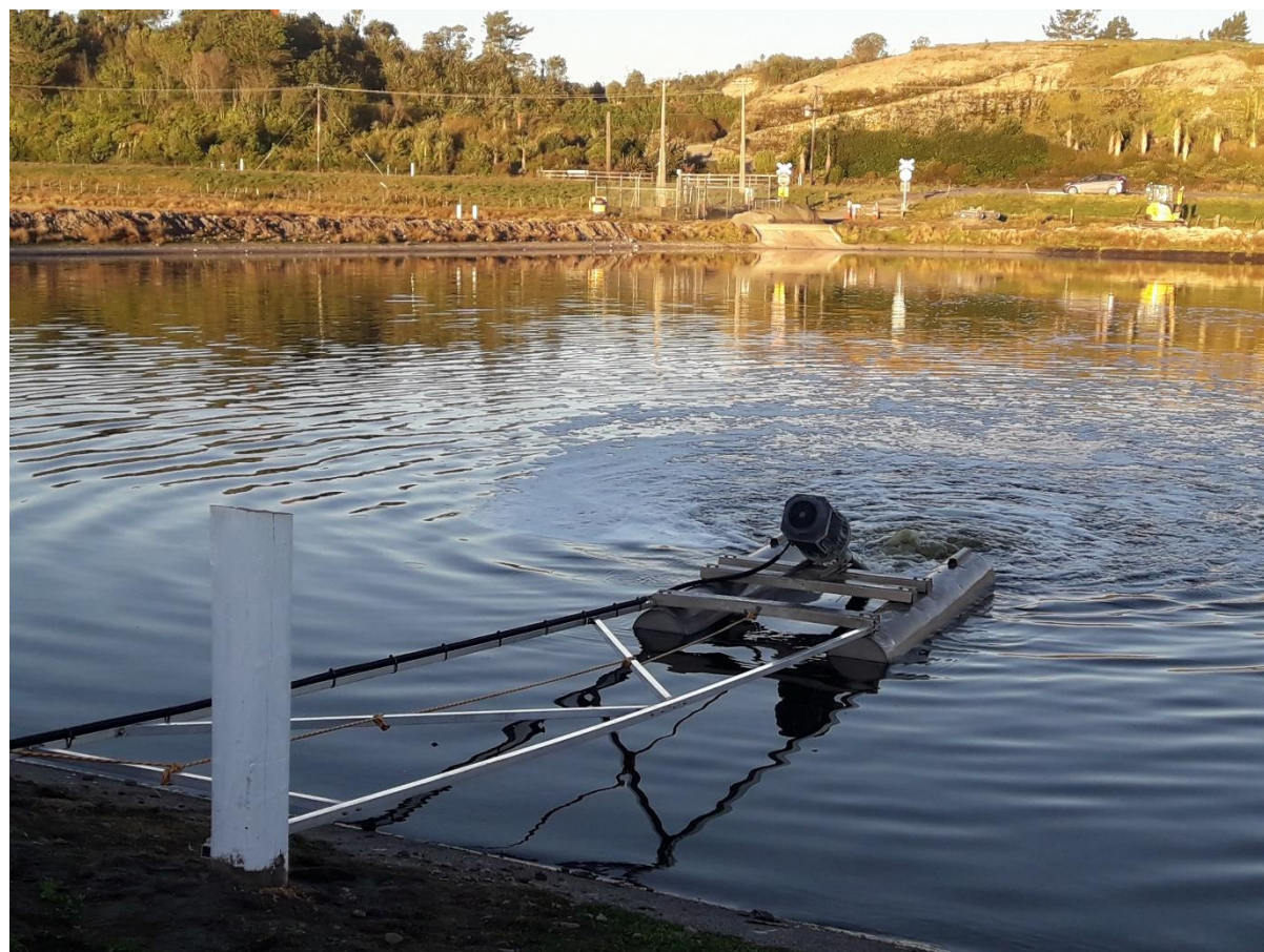
Image is one of the new aerators installed at the Hokitika Wastewater Oxidation Ponds during 2018 (Photo credit: M. Ross).
