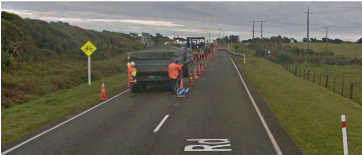
Warning sign – north of crossing
