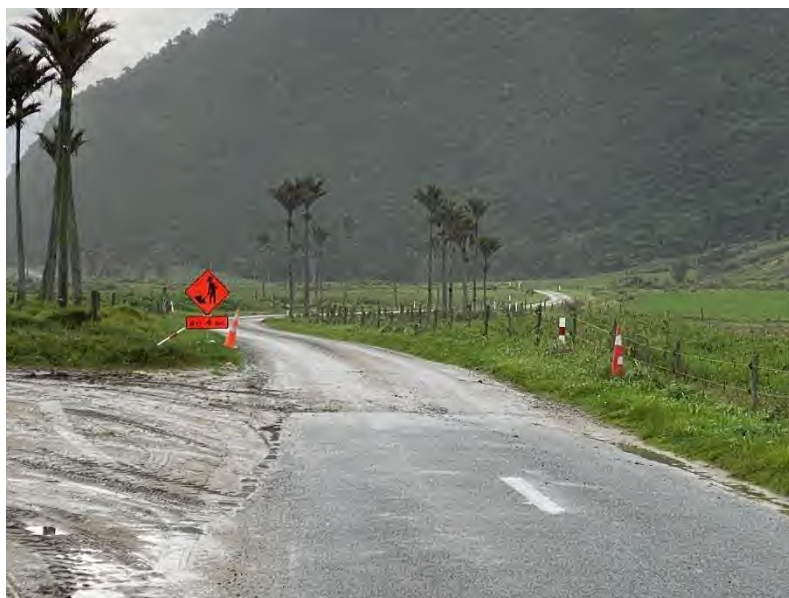
Figure 44: Karamea Highway – Kohaihai Road unsealed transition
