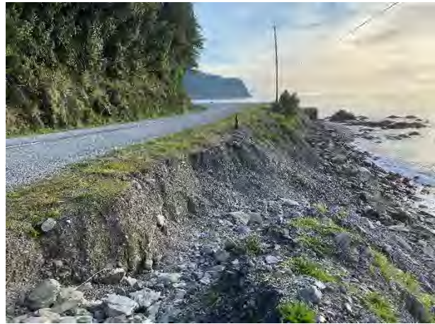
Figure 34: Coastal erosion at Jackson Bay, Westland District
