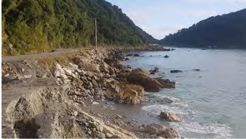
Figure 49: Coastal erosion and shoreline protection at Jackson Bay
