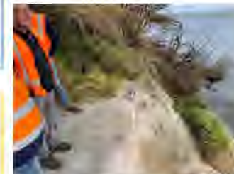
Okuru River Mouth erosion adjacent to road.
