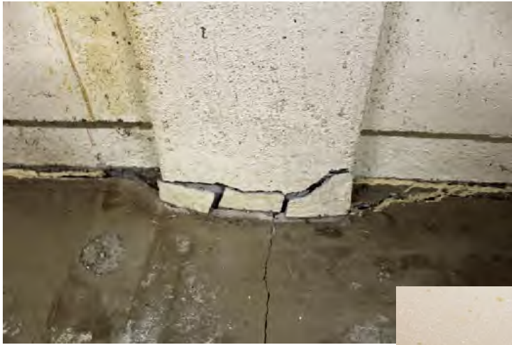
Cracking and subsidence between the walls, pillar and floor
