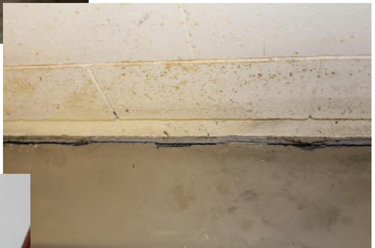
Cracking between the southern wall and floor
