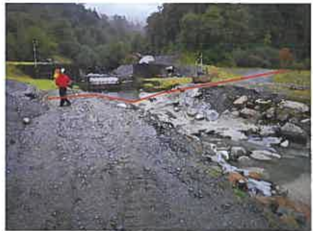
Figure 4: Weir AW3 crossing during Golder site inspection following remedial flood earthworks. Red line shows route of cycle track.
