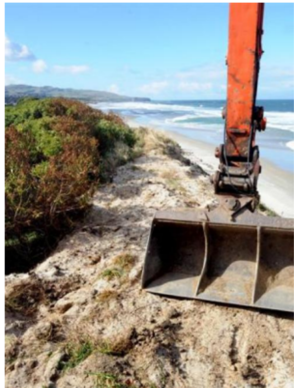
A digger works on top of the sand dunes at Middle Beach. Photo by Stephen Jaquiere.
