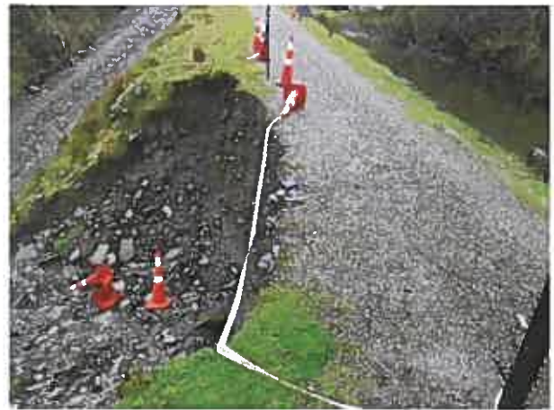
Figure 8: Flooding caused the diversion of river water behind an embankment that subsequently overtopped and eroded the downstream side. Photo west of Cowboy Paradise.
