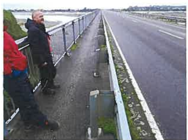
Figure 12: The Hokitika River bridge. Off road pathway is narrow and road safety barrier supports present a hazard to cyclists. Note that there is no shoulder width for cyclists on the road. Photo facing Hokitika.
