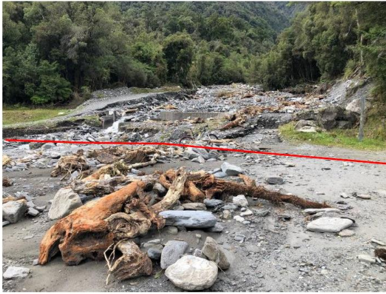
Figure 3: Weir AW2 crossing following March flood damage. Red line shows route of cycle track. Photo supplied by D. Inwood, dated 30 March 2019.
