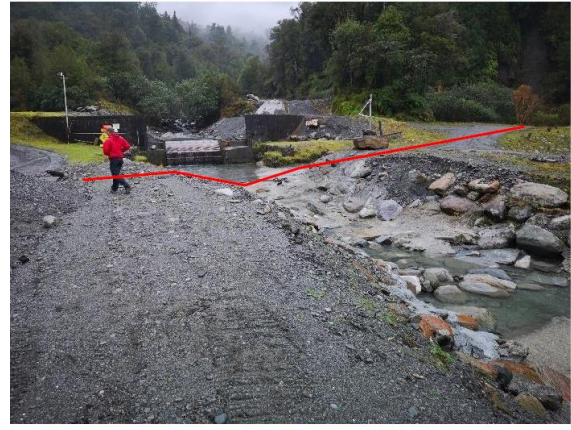
Figure 4: Weir AW3 crossing during Golder site inspection following remedial flood earthworks. Red line shows route of cycle track.
