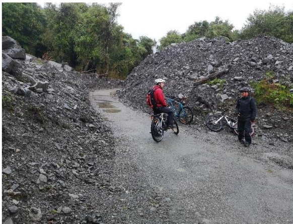
Figure 7: Recent clearing of a March 2019 debris flow to reopen cycle access. Debris flowed downhill from left to right. Photo west of Cowboy Paradise.
