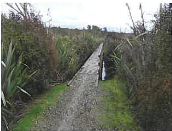
Figure 11: Example of a DoC bridge near Lake Mahinapua where transition narrows and hazards to cyclists from end of hand railing and potential drop into water either side of track.
