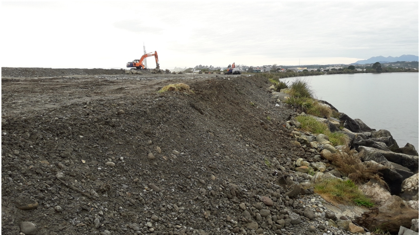
Raised fill protection prior to rock being placed on the river side
