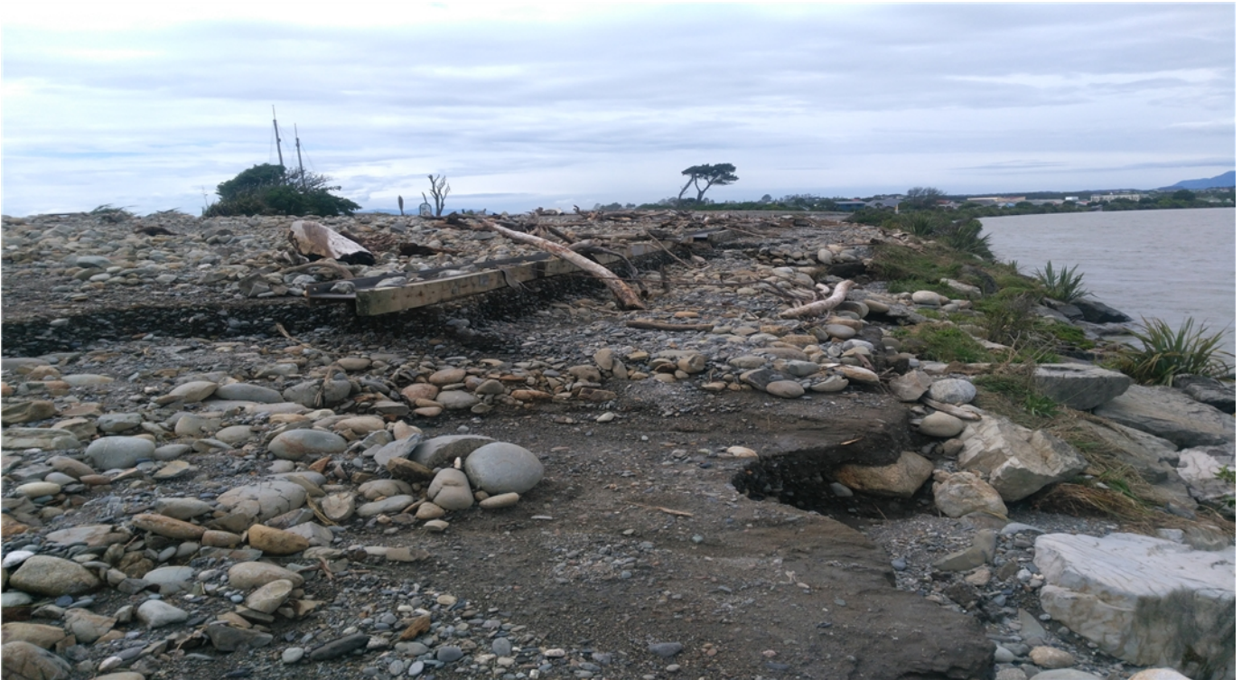
River side storm damage
