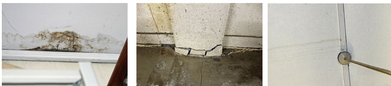
Leaks and cracking in the archive storage facilities.
