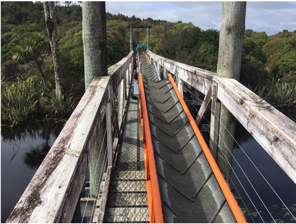
Conveyor Belts on DoC walkway bridge
