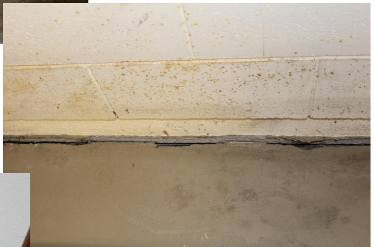
Cracking between the southern wall and floor
